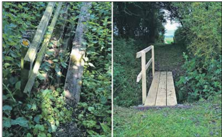
The collapsing footbridge (left) was replaced with a new bridge (right) after a Parish Path Warden reported the issue to the county council. Photos: Dave Cavanagh
