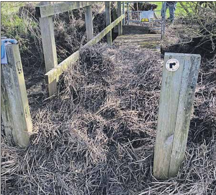
The footbridge at Felmersham before RIPPLE volunteers got to work. Photos: Steve Woodward
